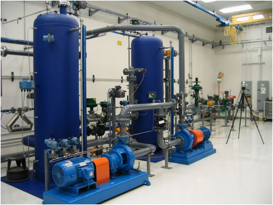
Figure 2.2 Performance Test Loop
