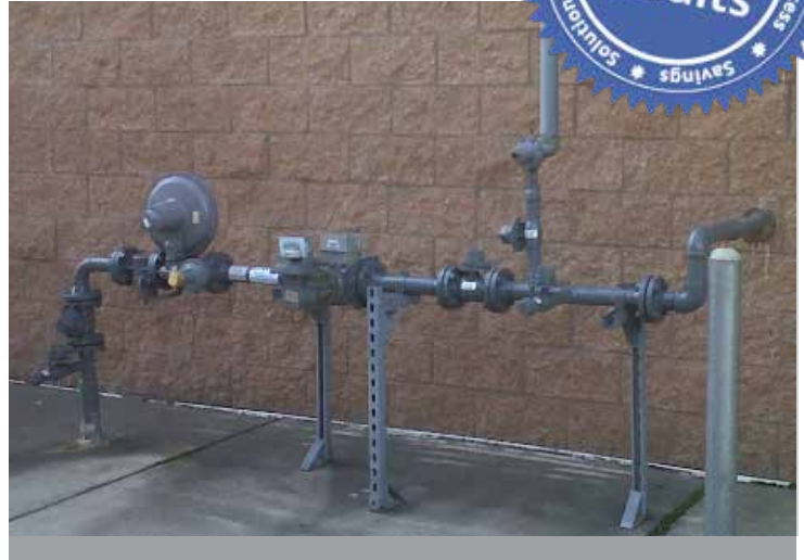
Existing regulator with secondary relief and vent stack downstream of the regulator.
