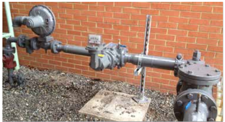
CS800IQ with high capacity relief eliminated the need for secondary overpressure protection device.
