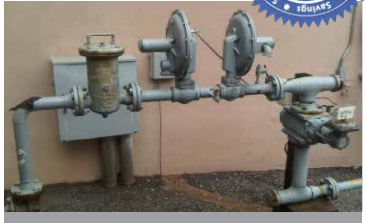
Traditional wide-open monitor arrangement with two regulators and external control line.
